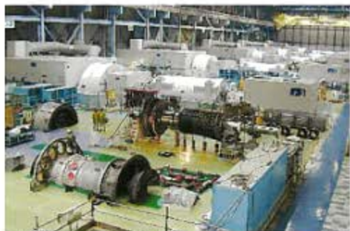
Periodic inspection of gas turbine at Shin-Nagoya Thermal Power Station
