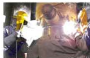
Welding work subject to inspection by welding operator under Electricity Business Act
