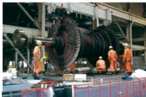
Periodic inspection of steam turbine at Hekinan Thermal Power Station
